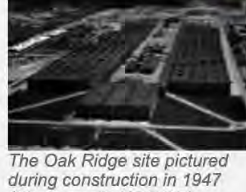
The Oak Ridge site pictured during construction in 1947 (Photo credit: US DOE)
